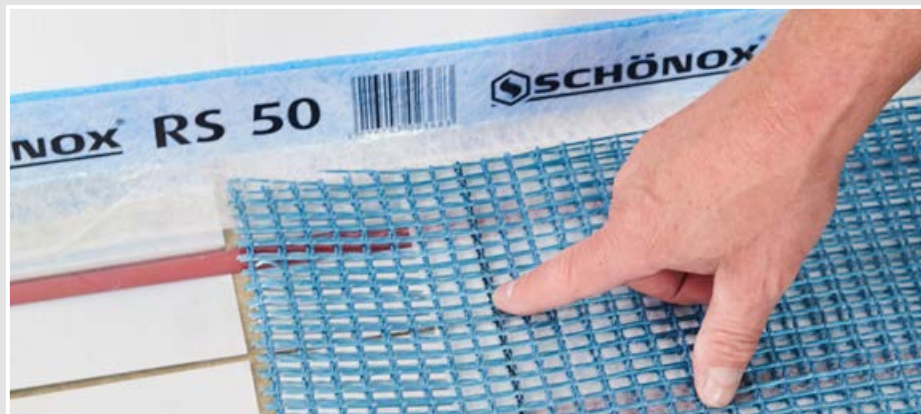
7 The fleece-backing has a recess of approx. 9 cm on one side. Place the side with the recess upwards, so that the levelling compound can run through.
