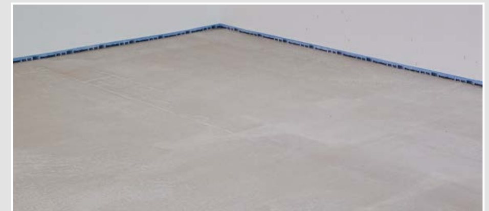
13 After 48 hours, the system is ready for the application of desired floor covering.
