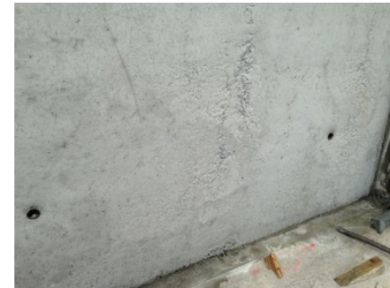
Extensive shrinkage cracks, surface blowholes and honeycombing must be repaired in advance
