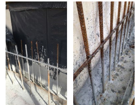
The protective sheet has served its purpose (photo left); Contamination should be avoided or be cleaned off immediately while still fresh (negative example pictured right)
