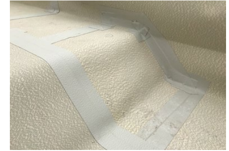
Non-standard corner detailing in a sloping area
