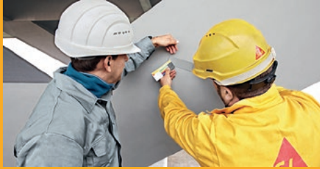
CORROSION AND FIRE PROTECTION
